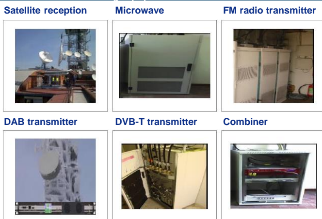
Rai Way – State-of-the-art broadcasting equipment
